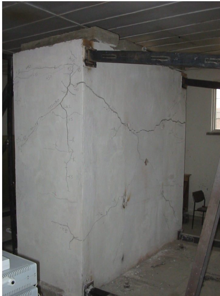
Figure 14. The cracks occurred at the front face of MW under out of plane cycling load.
