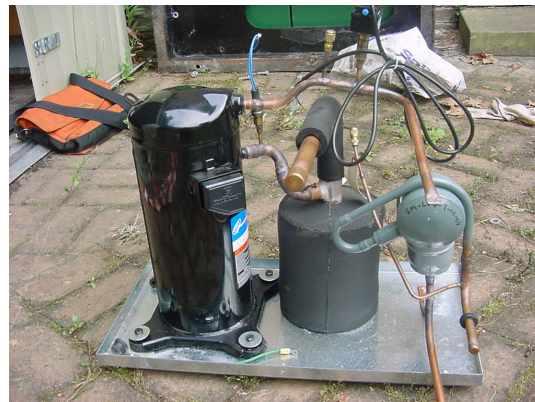
Figure 13. A photograph showing the connection of heat pump to the ground source.
