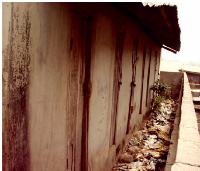
Figure 2. The rear side of the public toilet being used as a refuse dump.
