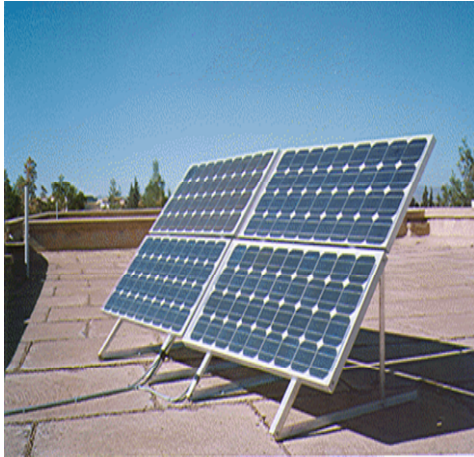
Figure 12. Photovoltaic panels SP75 installed in laboratory.
